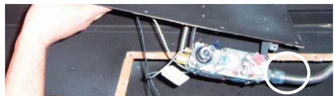
Gas Inlet Line
