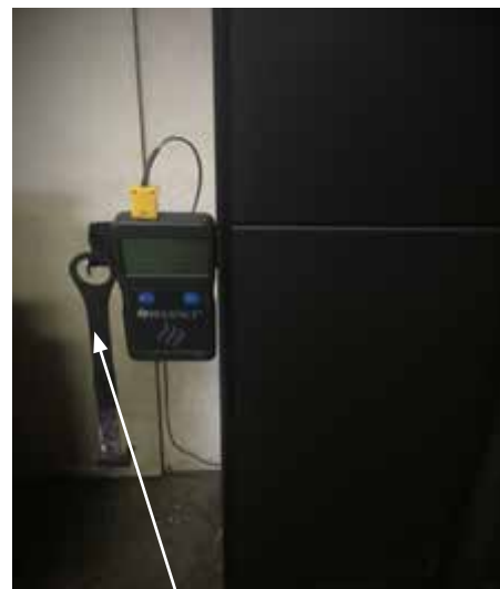
Air and Bypass operating handle/monitor storage.
