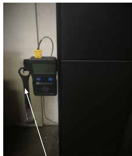
Air and Bypass operating handle/monitor storage.
