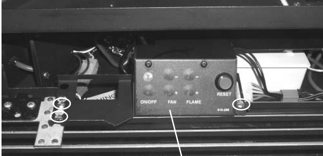
Manual Control Box
