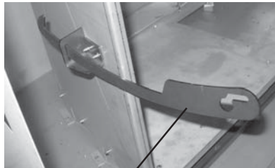
Hinge with door removed.
