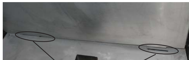
Slots on floor of firebox base.
