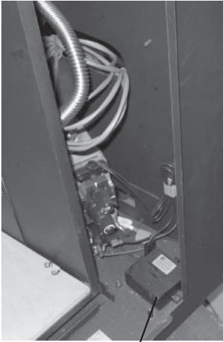
DC Spark Box Location
