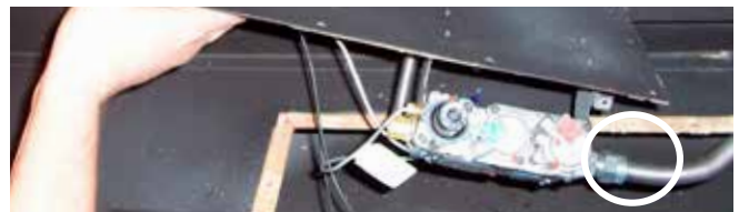
Gas Inlet Line
