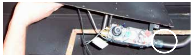
Gas Inlet Line
