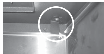
Bracket shown in place on right side of the firebox
