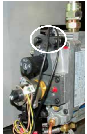
DC Sparker Wires
