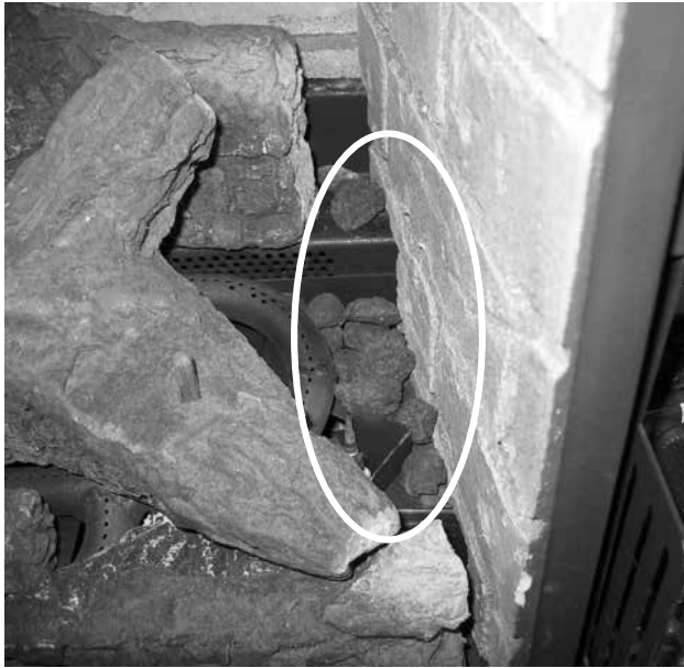
Right side of Burner
