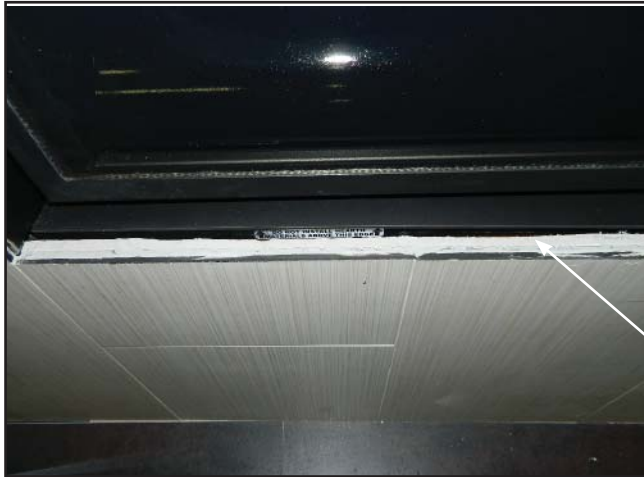
Figure 103 Top View - exposed non combustible materials
