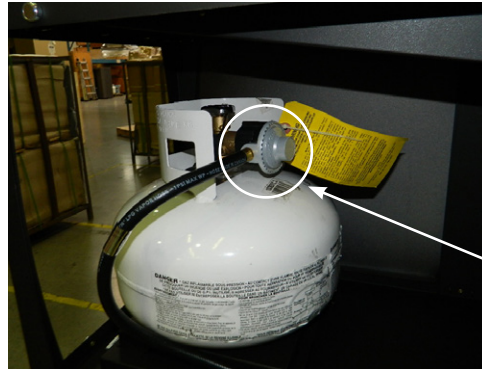
Gas connection @ tank
