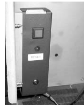
Located on the left hand side of the firebox behind the exterior brick panel.
