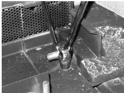
Burner Orifice Removal
