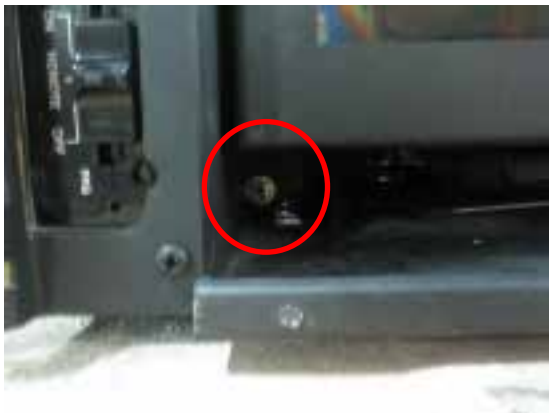
The Surefire switch is located at the bottom left corner of the unit.
