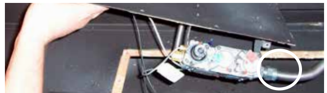
Gas Inlet Line
