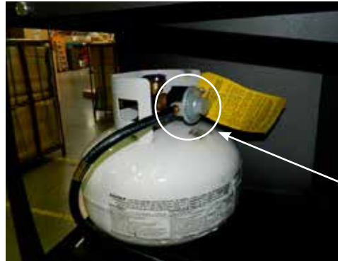
Gas connection @ tank
