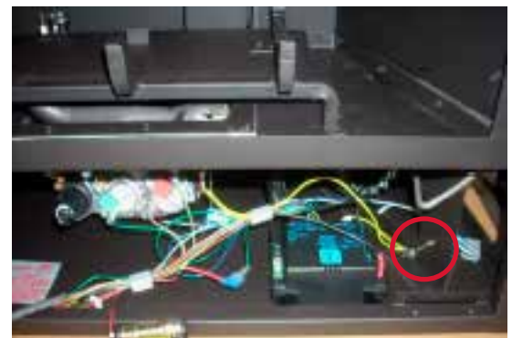
The Surefire switch is located in the bottom right corner of the bottom louver/panel.
