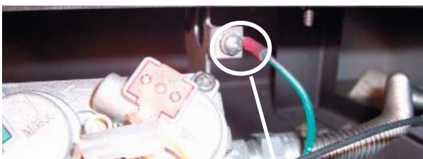
Green ground wire
