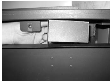
DC Spark Box Bracket Assembly partially removed.
