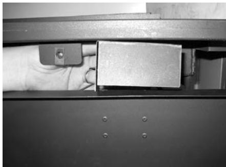
DC Spark Box Bracket Assembly partially removed.
