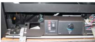
Burner ON/OFF control box attached to bottom flush louver.
