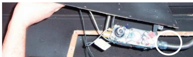
Gas Inlet Line
