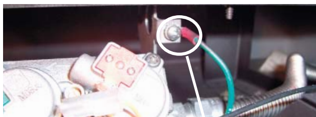
Green ground wire
