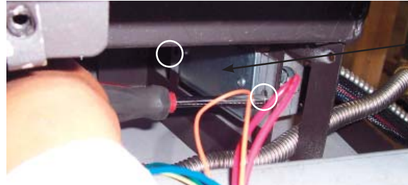
Electrical Box (Right side of Unit)
