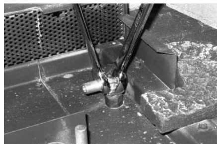
Burner Orifice Removal
