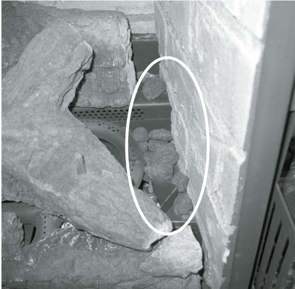
Right side of Burner
