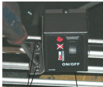
Screws on louver bracket Burner ON/OFF control box
